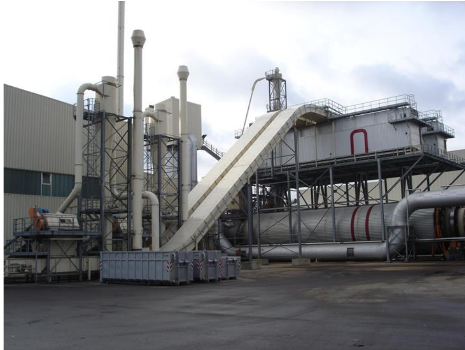
Figure 8 Single pass dryer in an OSB manufacturing process
